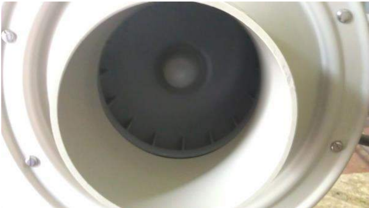
Room 3 – Extract Fan – Post Clean
