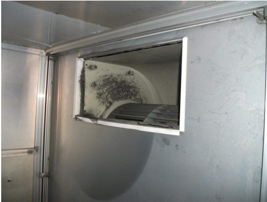
AHU025 Pre Clean
