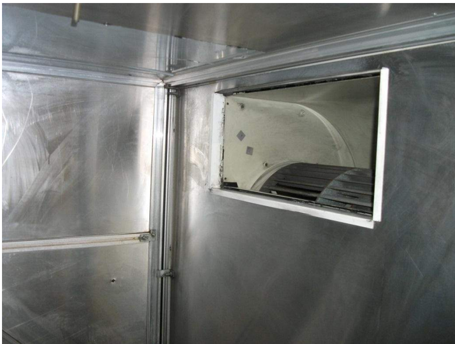
AHU025 Post Clean
